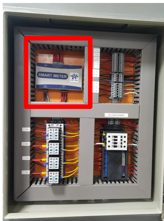
Figure 12 - Power distribution board where smart energy meter is installed - IoT Research Group Lab (Inatel).
