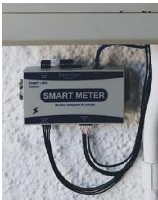
Figure 19 - Smart energy meter installed on TSDA Company three phase frame.
